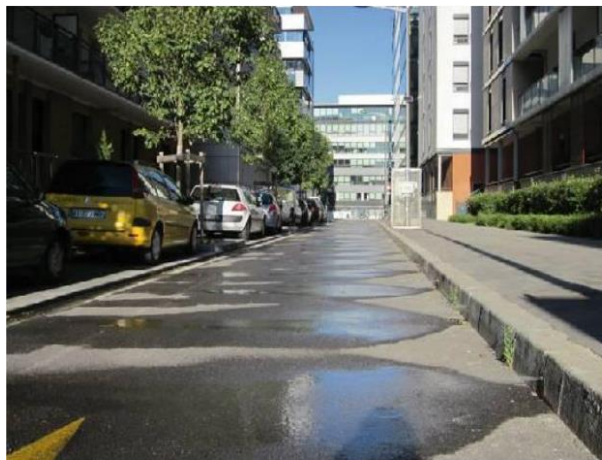
Fig a. Pavement watering device included in the curbside of the Buire street.
